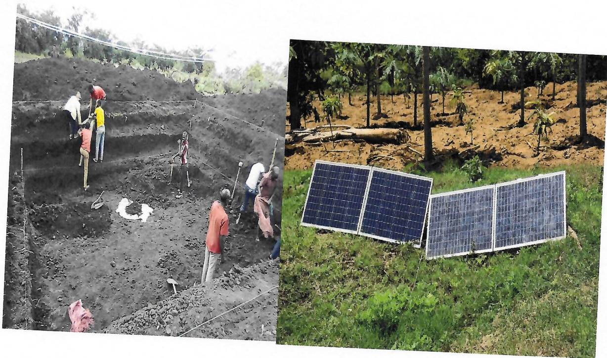
Fig 6 Pond construction ( in Doba woreda) and small scale irrigation development using solar water pump (in Gursum)
