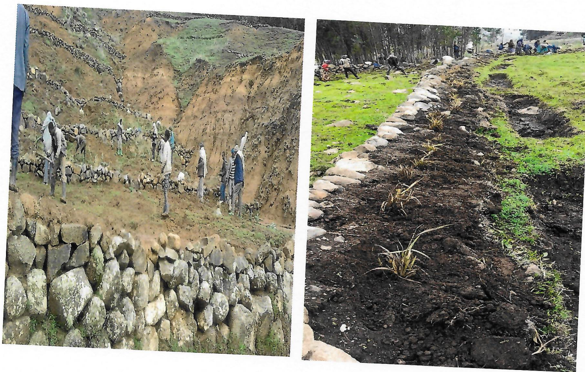
Fig 2 Construction of soil and water conservation structure and seedling production in Angolelana tera woreda
